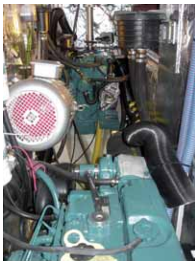
Trial engine and generator layout
