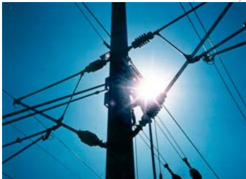
Overhead Contact Line OCL
